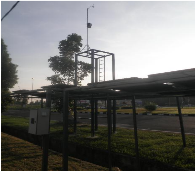
Fig. 2 Weather station and PV array
