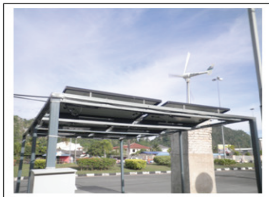
(b) PV array and wind power generation
